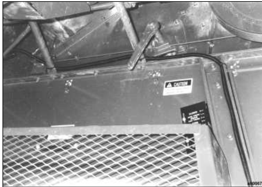
Figure 6. Elevator speed cable routed above rotor access door
